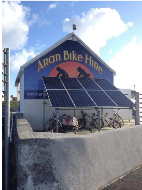
Solar PV at Aran Bike Hire, Aran Islands Energy Co-operative, Aran Islands
